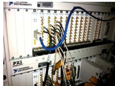
More than 200 AD channels in an expandable, customizable, rack system.
